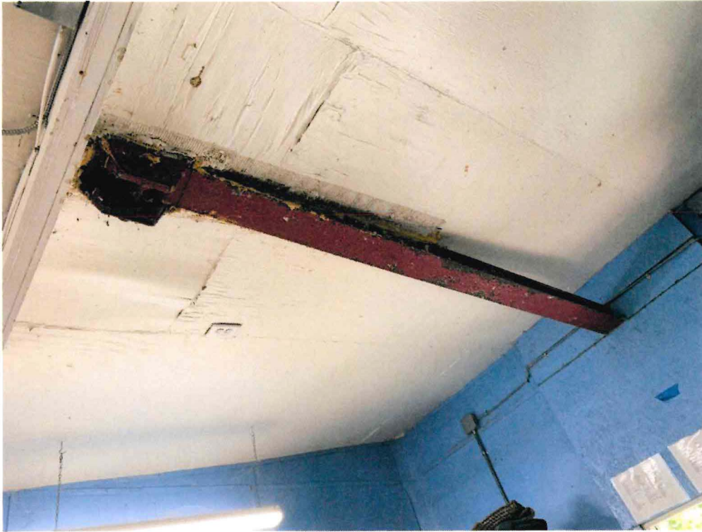
Lead Paint-Pole Barn
