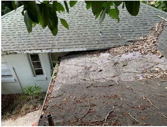
Problematic Front Entry
