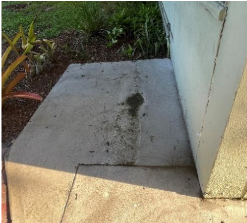
Pavement behind the restaurant affected by the lack of gutters on that side.
