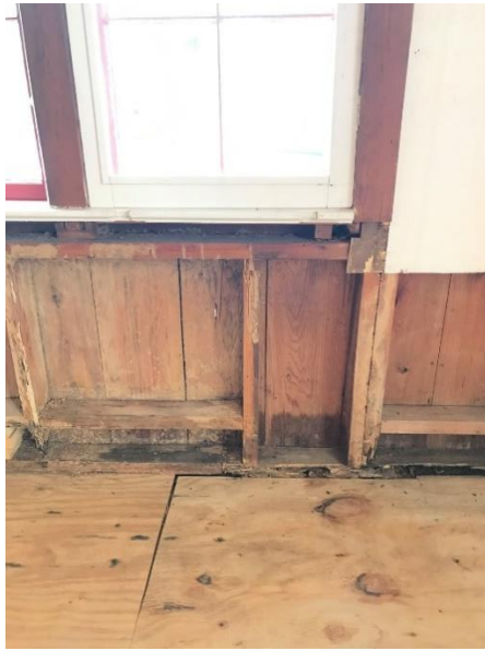
Close up termite damage
