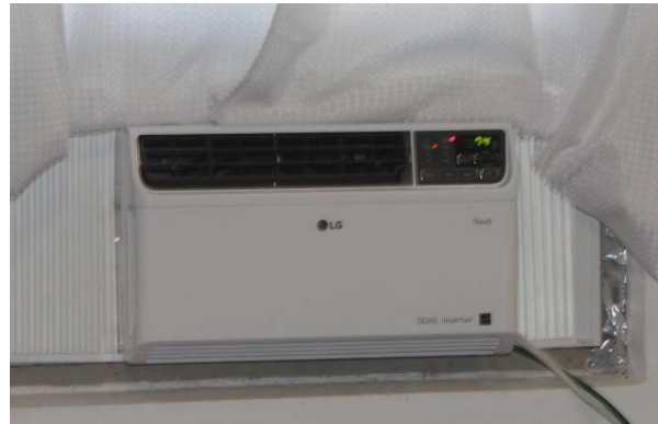
Through Wall A/C Unit
