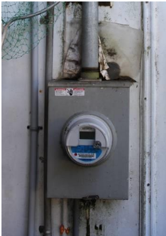
Barn service meter
