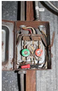
Maintenance shed fusebox
