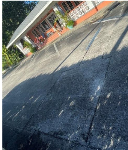
Large concrete patch
