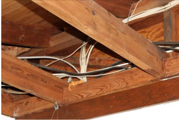
Exposed NM cable inside gift shop
