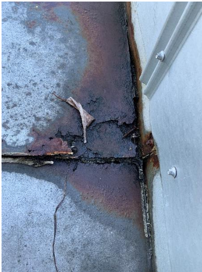
Corrosion at Storefront Valley
