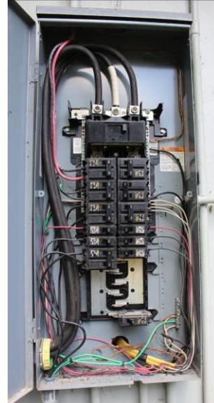
Electrical panel, cover removed
