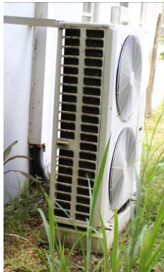
VRF Condensing Unit
