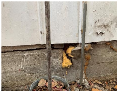
Deteriorated Foundation – North Wall Outside
