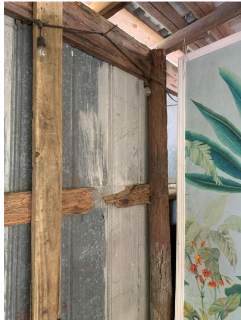
Wall Board Completely Failed
