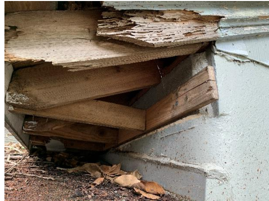
Front Entry Soffit Deterioration
