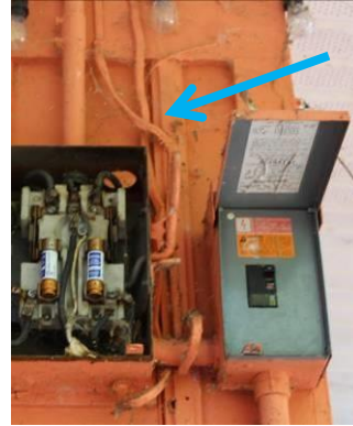
Exposed NM cable on exterior of gift shop
