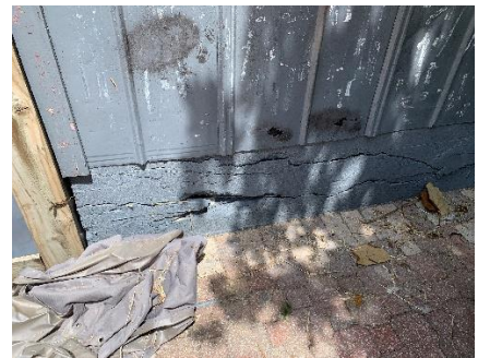
Deteriorated Foundation – North Wall Inside
