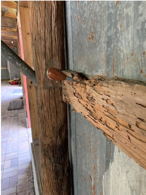
Heavily Deteriorated Wall Board
