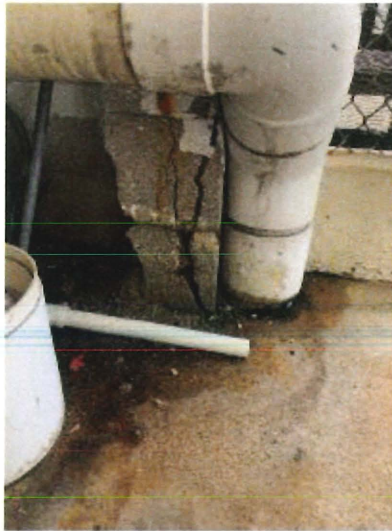
Base of CMU Column – Severe Corrosion
