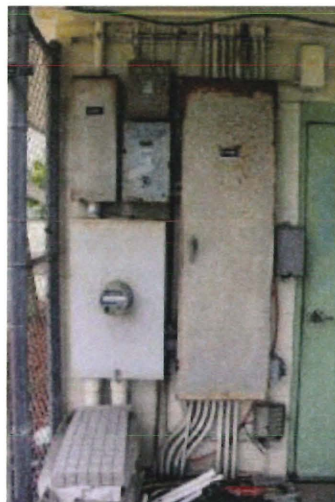
Electrical service equipment with pool tile
