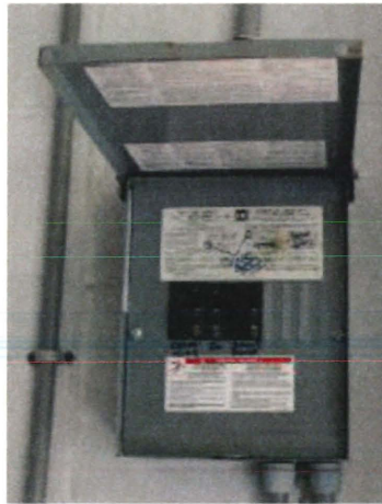
Panel "Subpanel A"
