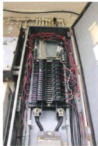
Panel "B" branch breakers
