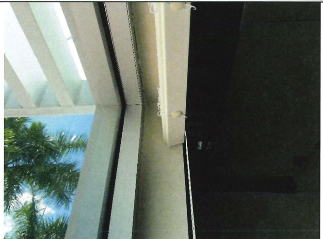
Photo 8: Assistant City Manager 222-Various cracks were observed on the inner window drywall.
