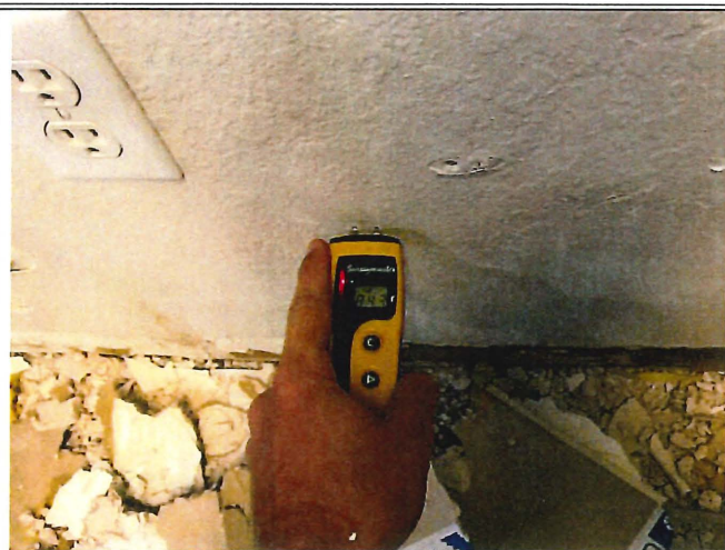
Photo 26: Reception 102 – Elevated moisture was detected in the drywall (84.3% WME).
