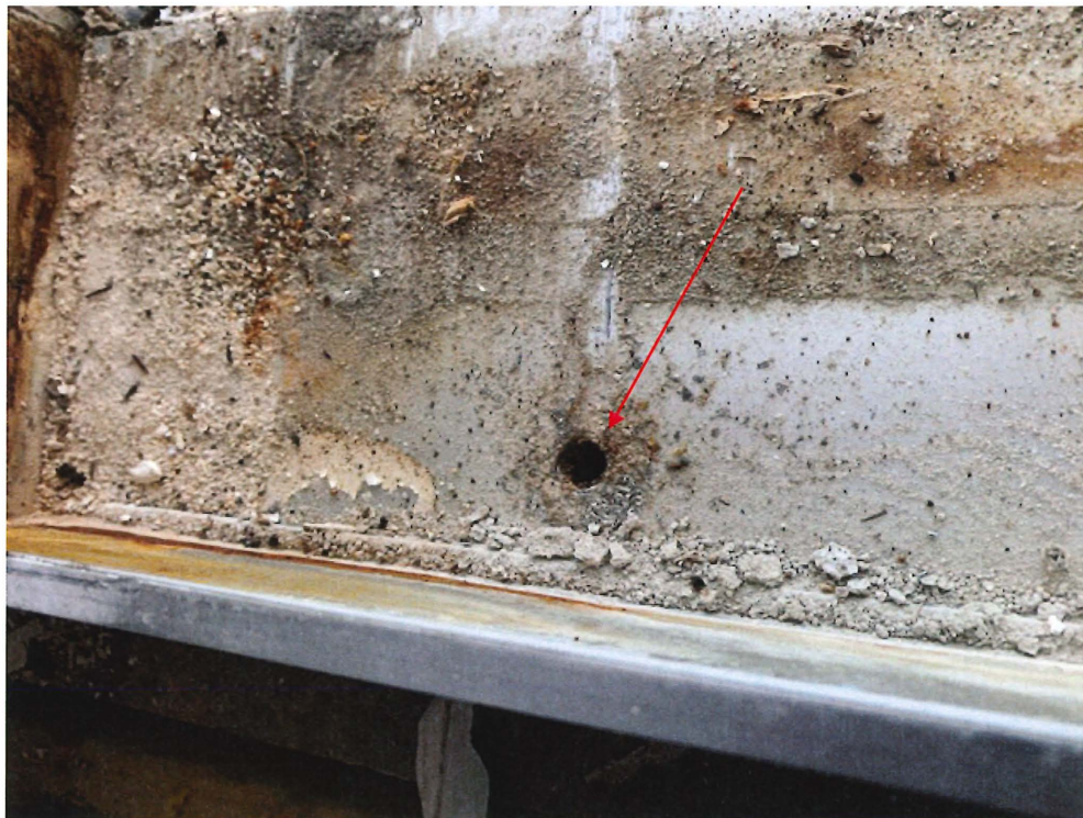
UNSEALED ANCHOR PENETRATION AT SILL FLASHING
