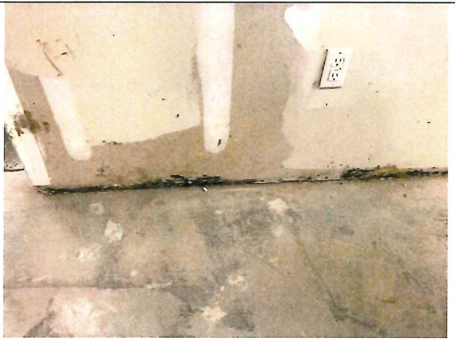
Photo 16: Mechanical Room 116 – Visible suspect mold growth was observed on the right wall up approximately eight-feet (8') around the outdoor vents and on all other walls.
