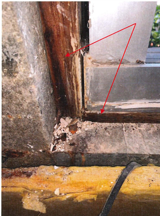
ROTTEN WOOD BLOCKING AT JAMB/SILL
