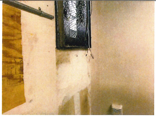
Photo 14: Mechanical Room 116 – Visible suspect mold growth was observed on the right wall up approximately eight-feet (8') around the outdoor vents and on all other walls.
