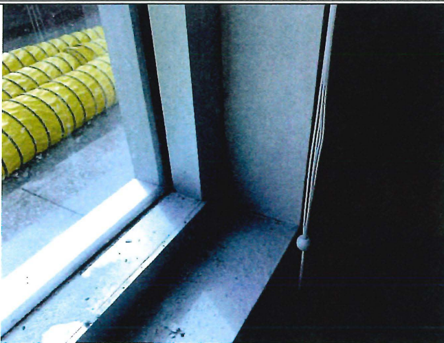
Photo 7: Break Room - Water damage was observed on the drywall and caulking around the window.
