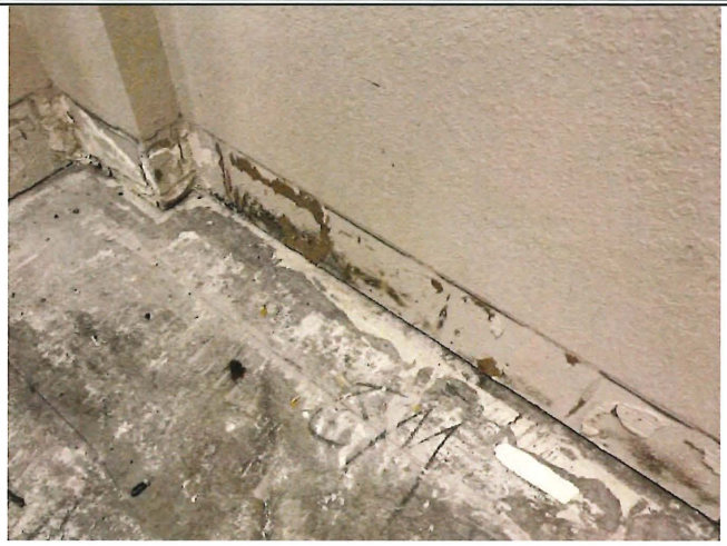
Photo 12: Stair 201A/Vestibule201/Adjacent Cubicles- Visible suspect mold growth was observed at the base of the drywall where the cove base had been removed.
