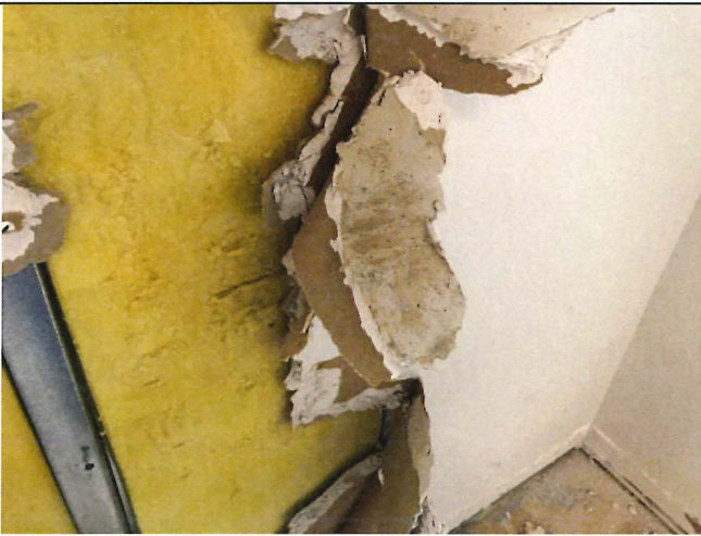
Photo 7: Assistant City Manager 222- Visible suspect mold growth was observed on the backside of the drywall.
