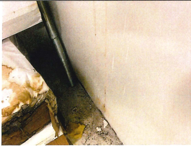
Photo 17: Mechanical Room 116 – Visible suspect mold growth was observed on the right wall up approximately eight-feet (8') around the outdoor vents and on all other walls.
