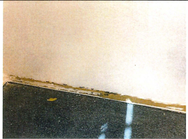
Photo 34: Office 106 - Visible suspect mold growth was observed on the front and left wall.
