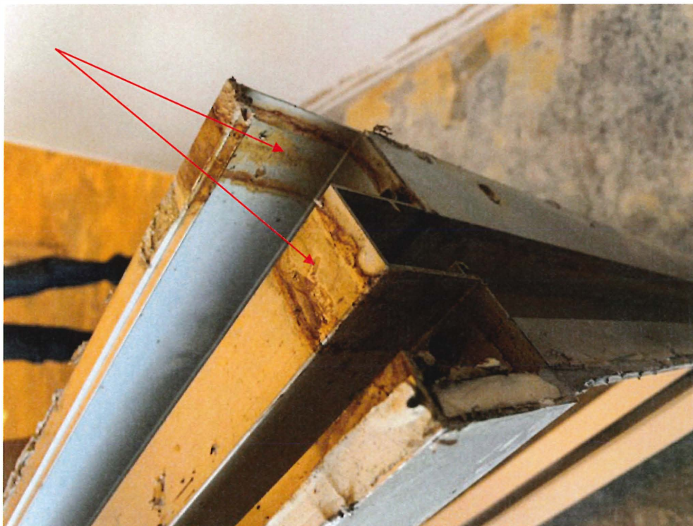
RESIDUE INDICATING WATER TRAPPED IN SYSTEM
