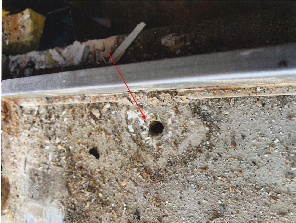
UNSEALED ANCHOR PENETRATION AT SILL FLASHING
