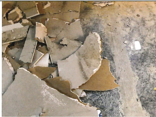
Photo 4: City Manager 220-Visible suspect mold growth was observed on the backside of the removed drywall.
