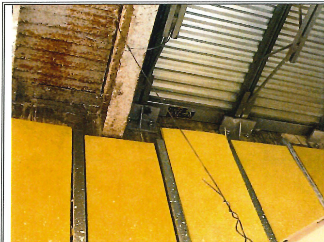
Photo 9: Break Room - Water staining was observed on the block near the ceiling.
