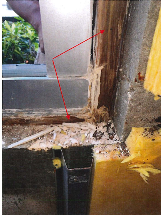
ROTTEN WOOD BLOCKING AT JAMB/SILL
