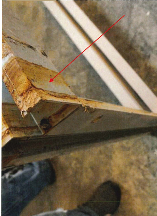
RESIDUE INDICATING WATER TRAPPED IN SYSTEM
