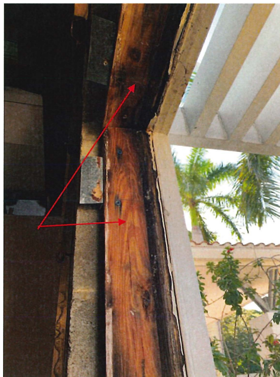
ROTTEN WOOD BLOCKING AT JAMB/HEAD
