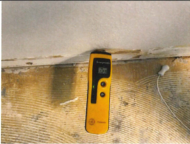
Photo 5: City Manager 220-Elevated moisture was not detected.
