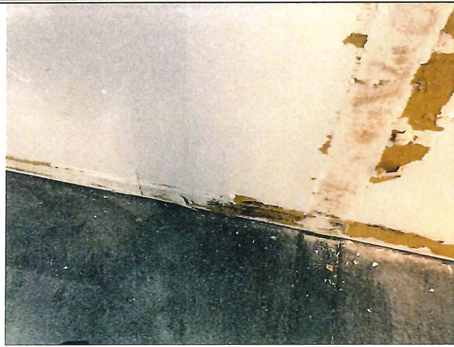
Photo 29: Office 105 – Visible suspect mold growth was observed on the front wall.
