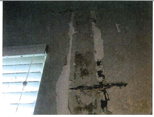
Photo 30: Office 105 – Visible suspect mold growth was observed on the front wall.
