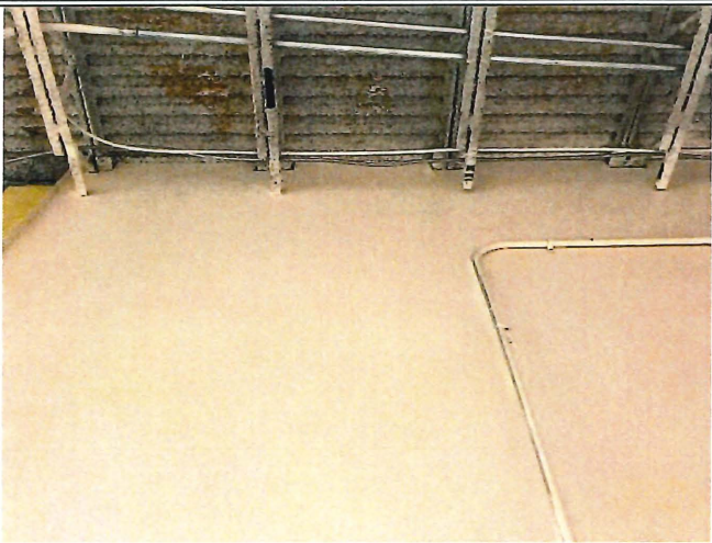
Photo 19: Mechanical Room 116 – Bubbling paint was observed on the right wall approximately ten-feet (10') up.
