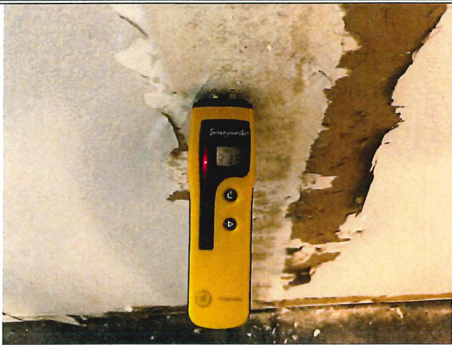
Photo 31: Office 105 – Elevated moisture was detected in the drywall (31.9% WME).
