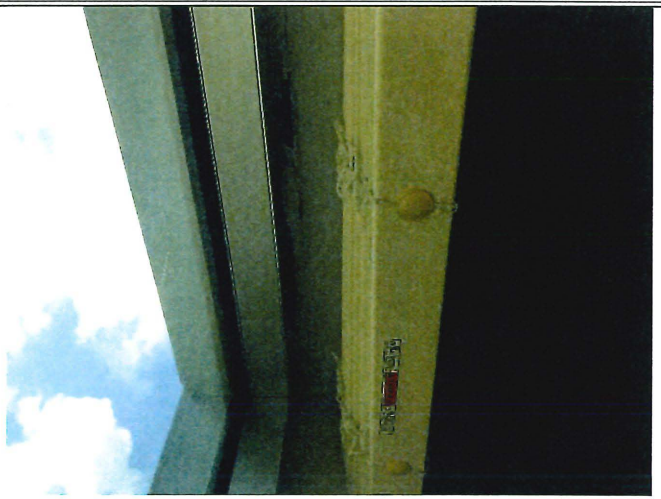
Photo 8: Break Room - Water damage was observed on the drywall and caulking around the window.
