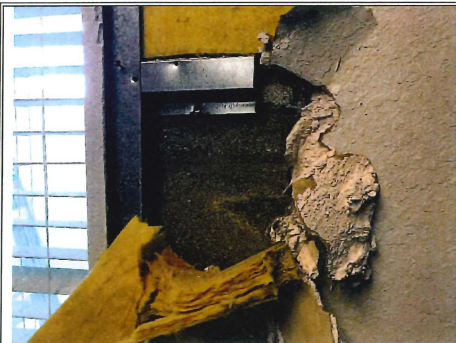
Photo 25: Reception 102 – Visible suspect mold growth was observed around the window.
