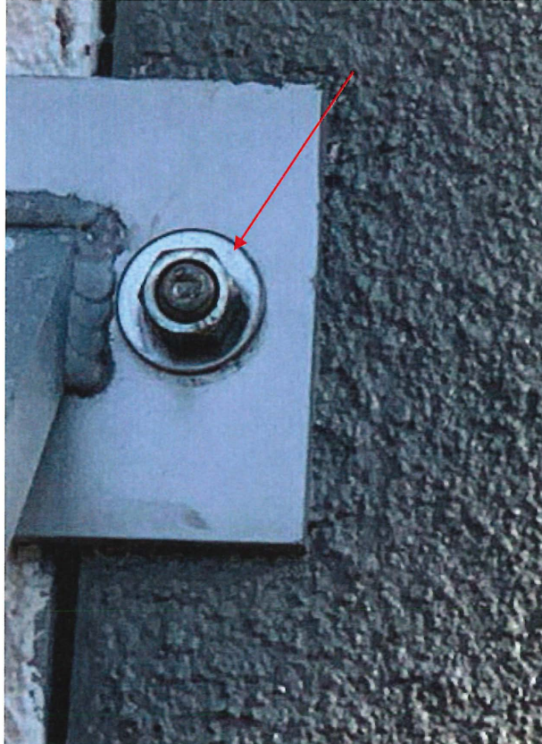
UNSEALED SUN SHADE ATTACHMENT ANCHORS
