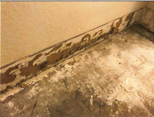
Photo 11: Stair 201A/Vestibule201/Adjacent Cubicles- Visible suspect mold growth was observed at the base of the drywall where the cove base had been removed.
