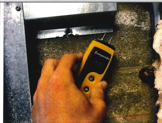
Photo 27: Reception 102 – Elevated moisture was detected in the block (999 REL).
