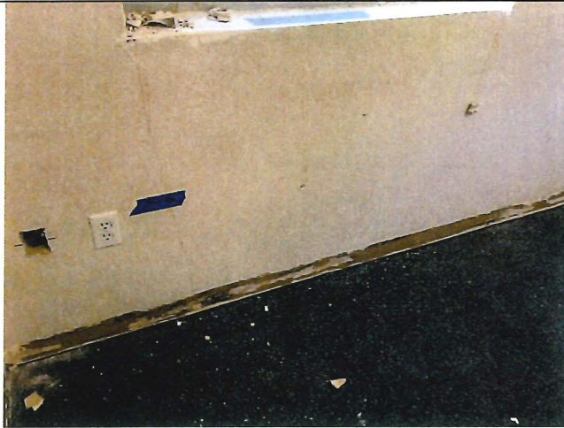
Photo 33: Office 106 - Visible suspect mold growth was observed on the front and left wall.
