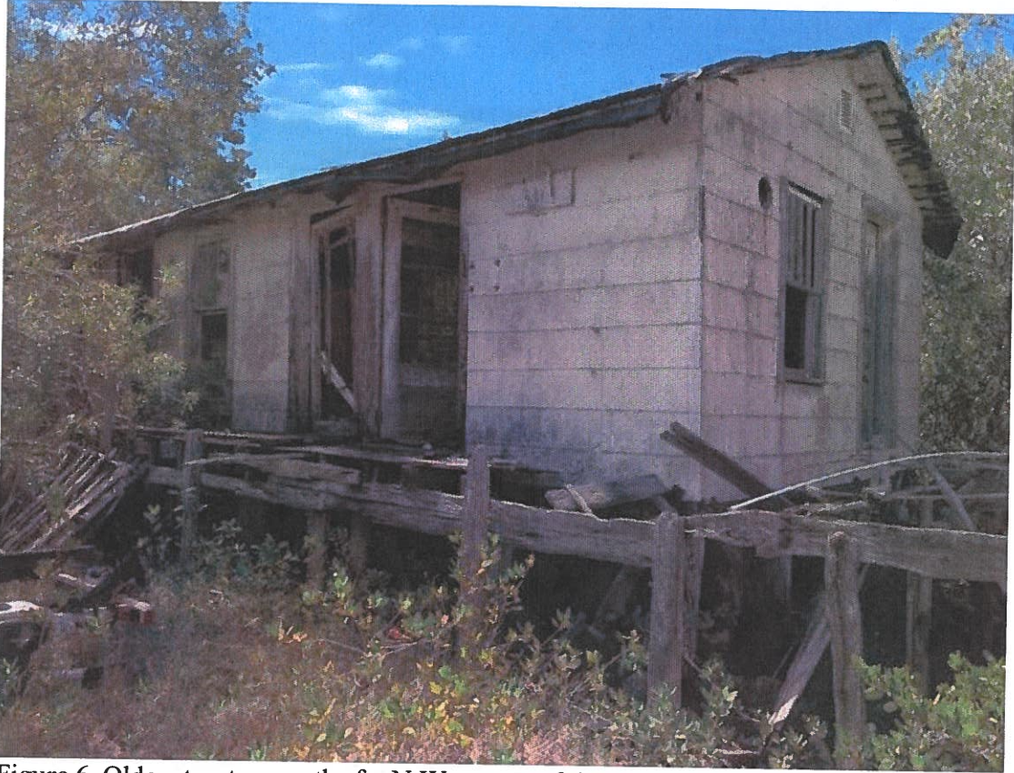
Figure 6. Older structure on the far N.W. corner of the parcel. The building is orientated roughly N-S, view looking S.W.
