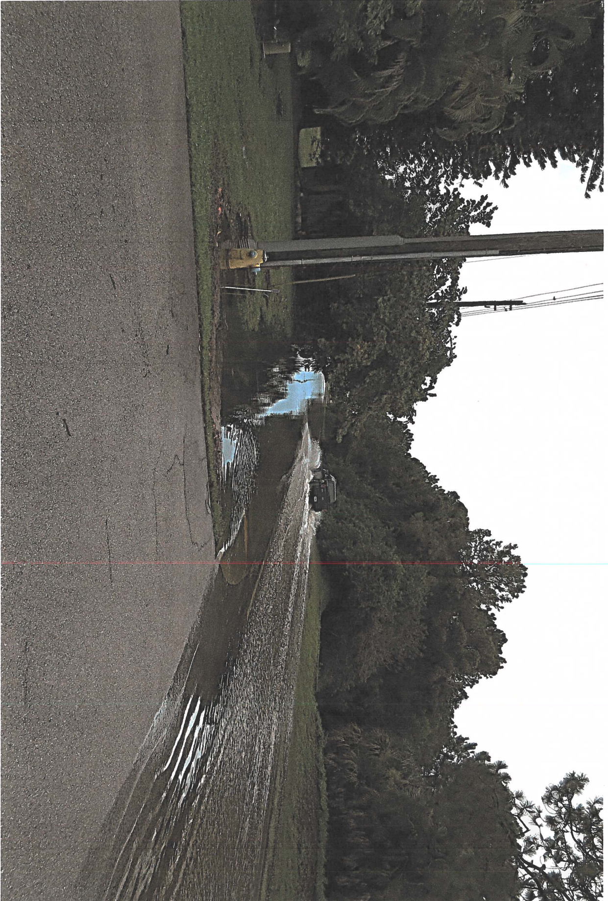
Cockleshell Drive at south entrance to Cypress Plantations 1 Condo Association. The car is passing over the culvert running under Cockleshell Drive. It moves water from a stream on the golf course to the Spring Creek. To the left of the car is a patch of wooden fencing under a tree where water pumping equipment was used in years past to drain flood water from the course. The wooden fencing was recently removed and replaced with chain link fencing. Photograph taken by Bonita Springs resident, John O'Brien on August 27, 2017.
