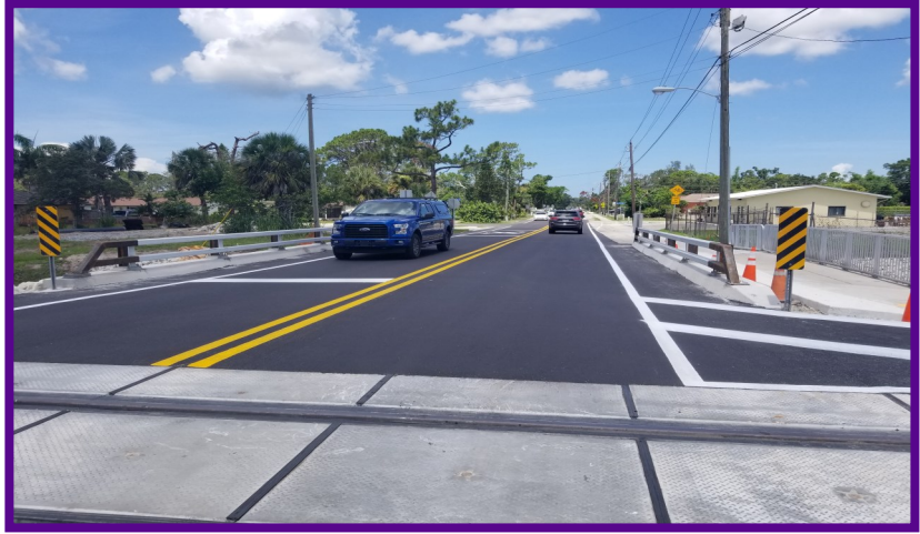
Photos left and above: Repairs are complete on the Terry Street Railroad crossings.
