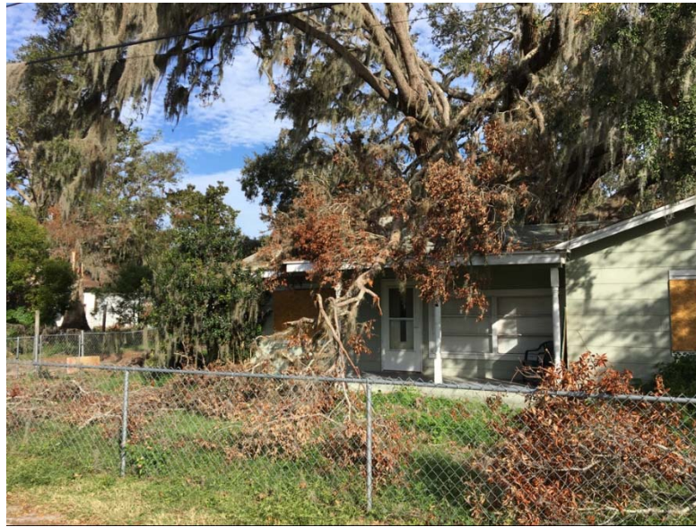
Tree damage and debris from recent high winds in Geiger Road area
