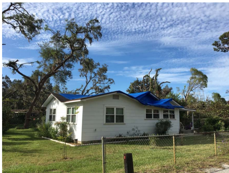
Wind caused roof damage Geiger Road area
